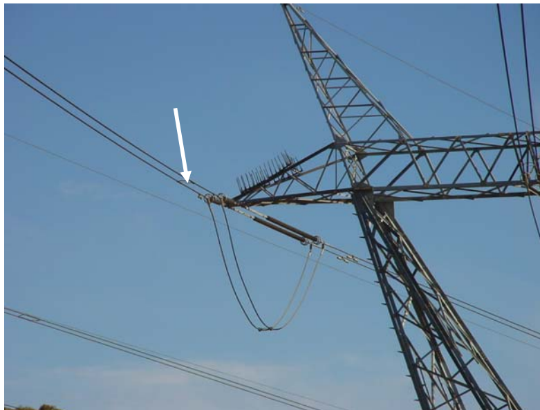
Picture of incorrect fitting leaving the landing plates exposed
